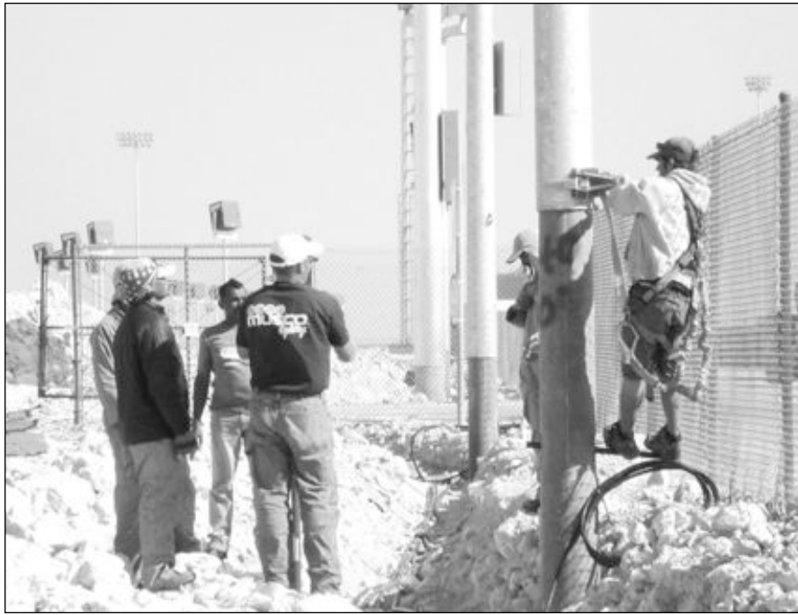
Musco Completes World's Largest Permanent Lighting Project: Musco members worked with an international team in extreme weather conditions to light the Losail International Circuit in Doha, Qatar. The project took 175 days, from design to install, and required drilling and trenching through 7.5 miles of rock to lay over 310 miles of wiring.
