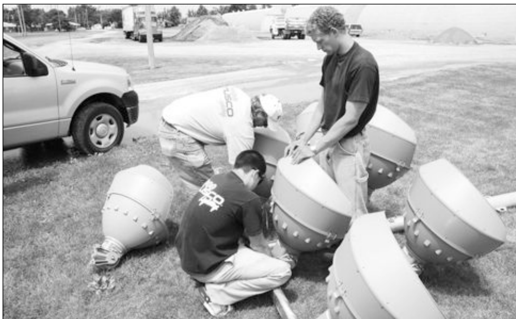
Team Install Help a Win/Win: Musco Team members assist area schools with volunteer installation to help cut project costs and to provide hands-on training for Musco members working with the product. Above, members assemble the New Sharon Little League system on-site.
